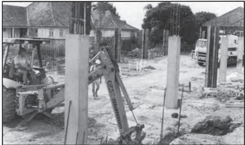
The Churchie contract involves four different sections, with the main section being a new multi-purpose block.
