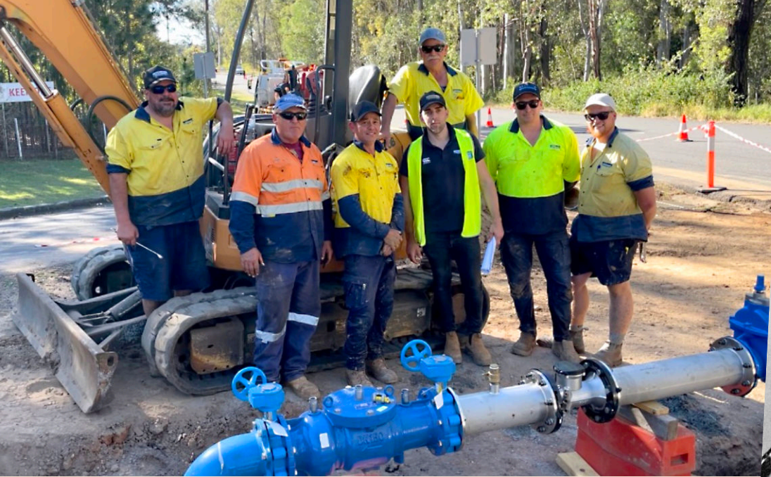
Some of Hutchies' plumbing team who recently carried out a live connection to a 300mm water main at Wacol correctional facility. It was a big job which risked water supply to hundreds of homes, but the work went off without a hitch.
