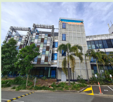
Hutchies' third remedial cladding project for Queensland Health was at Forensic and Scientific Services (FSS) campus at Coopers Plains.
