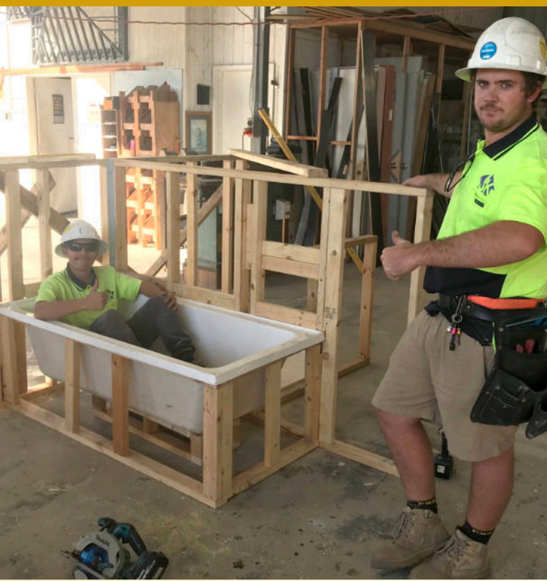
Duncan MacFarlane gives Harrison Smith the thumbs up to the bath tub installation following their wet area framing workshop. Duncan and Harrison work for J&K Constructions, a sub-contractor working at Hutchies' modular yard at Yatala.
