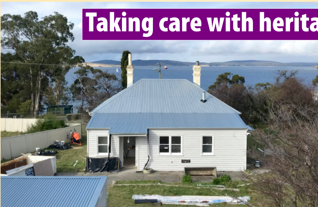
The finishing touches are put to the refurbished former caretaker's cottage for the University of Tasmania.
