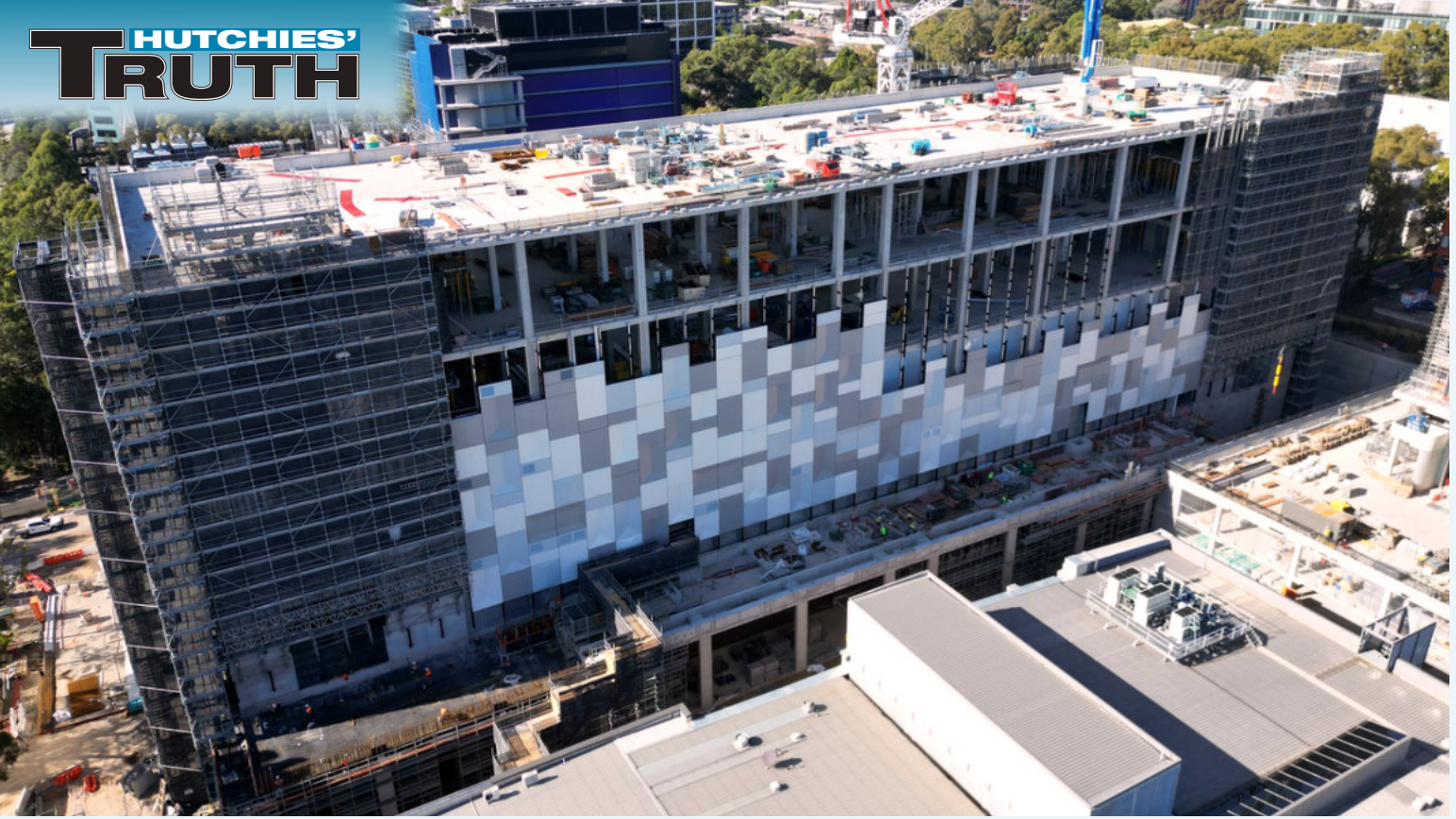
A new data centre is under construction at Macquarie Park in Sydney.
