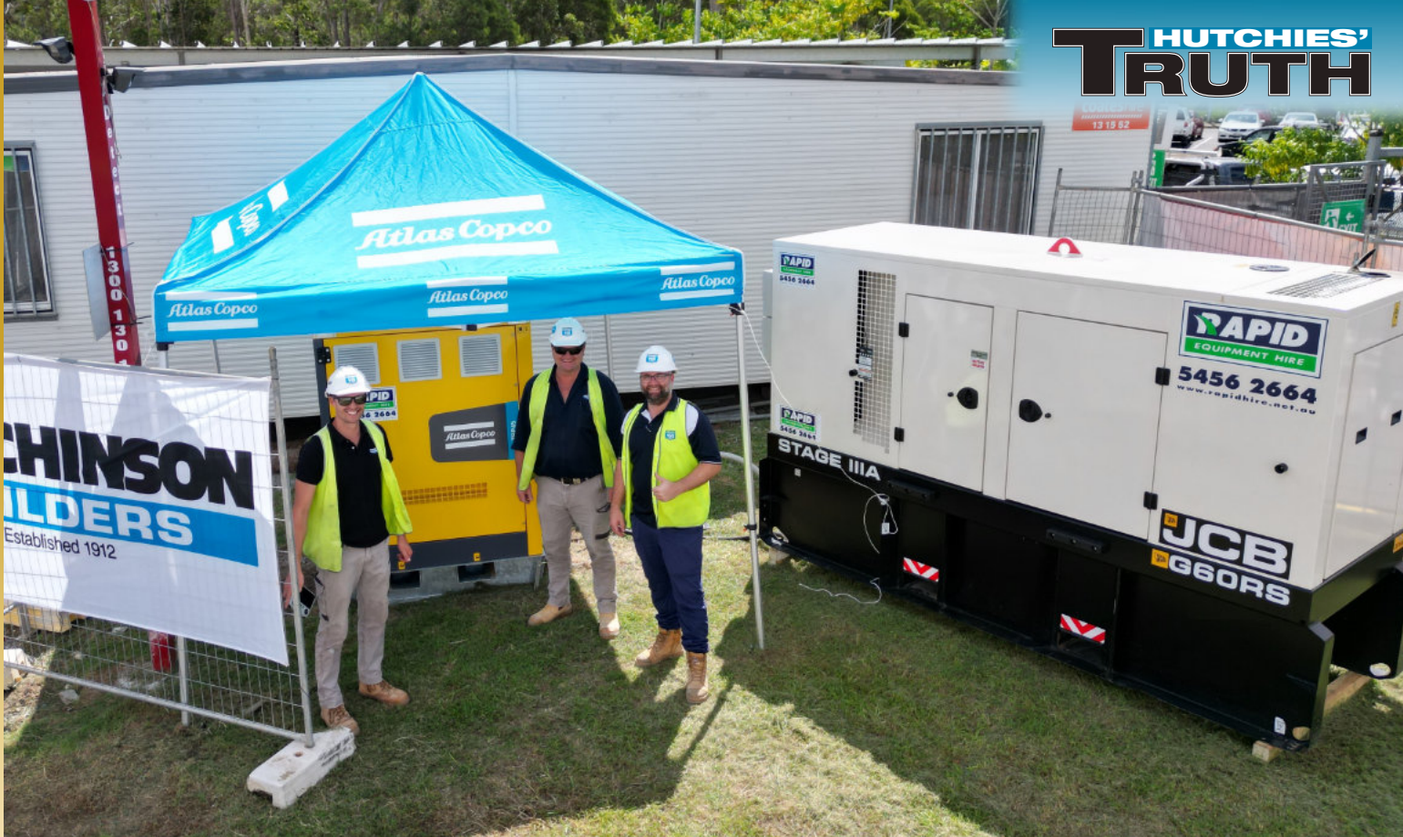
Hutchies' site team at Kallangur (from left), Shane Couchman, Wade McGrath and Nathan Byrne, with the new power set-up to reduce fuel load and emissions.
