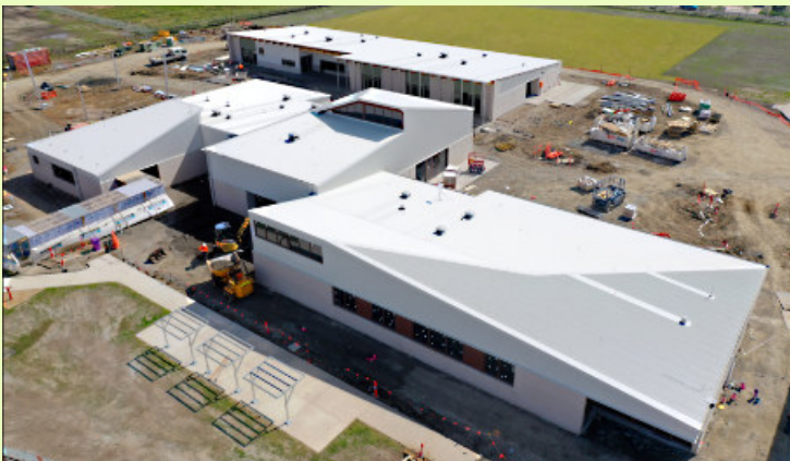
Yubup Primary School, one of six under construction by Hutchies for the Victorian School Building Authority.
