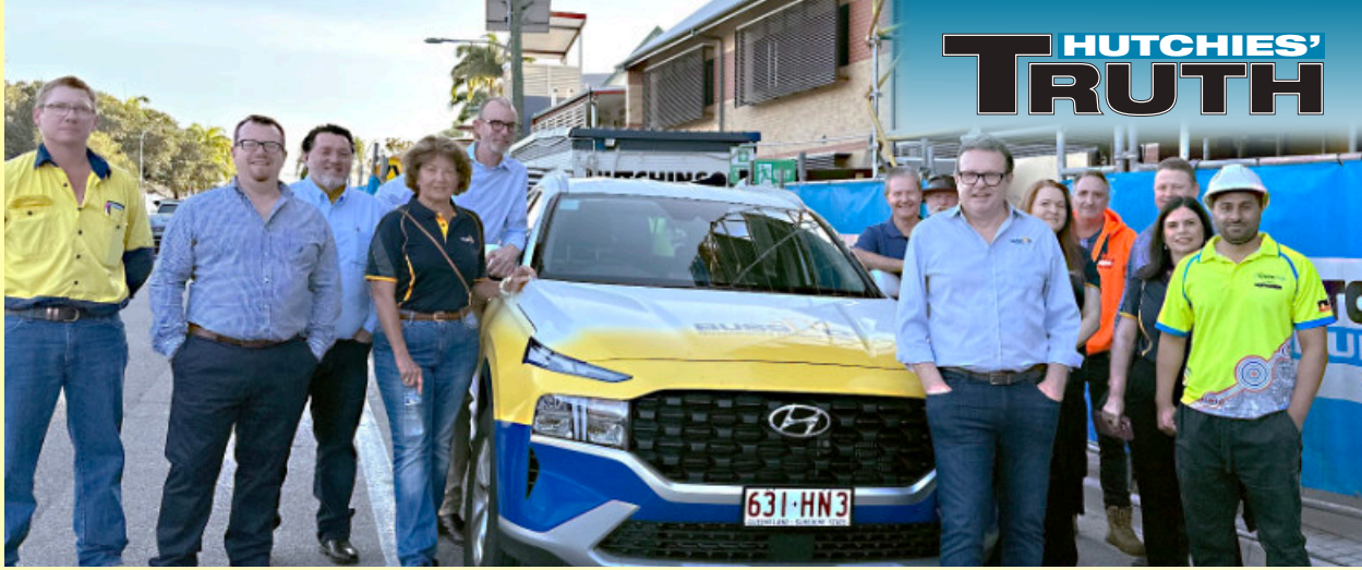
During their visit to Townsville, BUSSQ board and senior executives met with members of Hutchies' team on St Patrick's College project.
