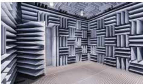
CSIRO Reverberation & Anechoic Chambers Clayton, VIC
